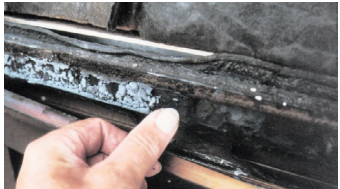
Figure 6: Residential building using silicone bonded glazing after external fire. The silicone shows a silica char.
