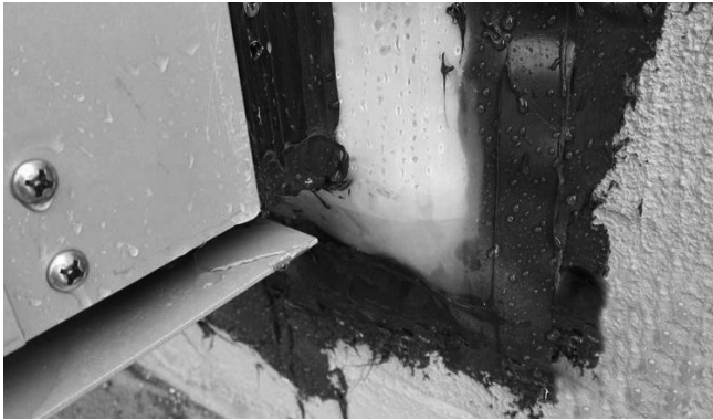
Figure 4: Sealant attaching strip and corner to air barrier in-field. Lap joints sealed.
